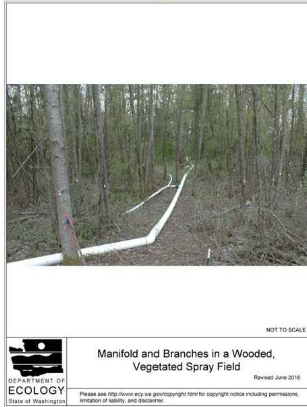
Figure II-3.25: Manifold and Branches in a Wooded, Vegetated Spray Field
